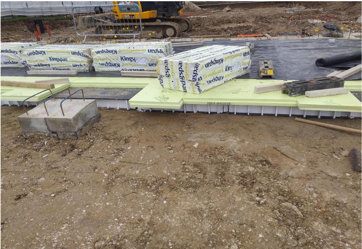
Top of pile cap exposed, 100mm cellcore to allow for heave and 80mm under slab insulation
