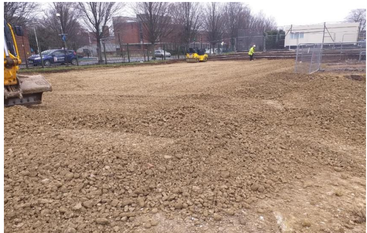
Piling mat being installed, 300mm of recycled 6F5 crushed stone, the piling mat must be strong enough to take the weight of the piling rig whilst it is drilling
