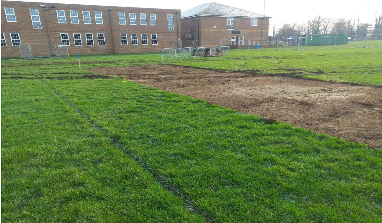
First buckets in the ground, vegetation is removed from site as waste but the topsoil is saved on site for future reinstatement
