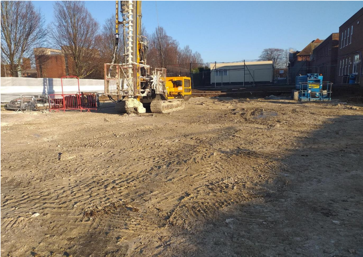
Piling rig in position, a total of 125 piles were drilled to depths ranging from 8m to 15m, reinforced steel added, concrete poured to give them strength
