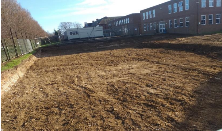
Excavation for the piling mat, we dig down to solid ground before building back up with stone for strength
