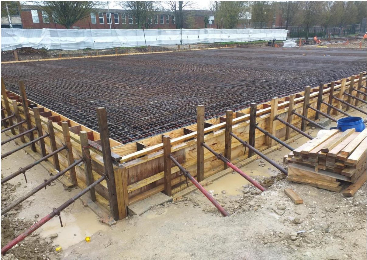
Reinforcement finished, timber shuttering in place to contain the concrete when it is poured
